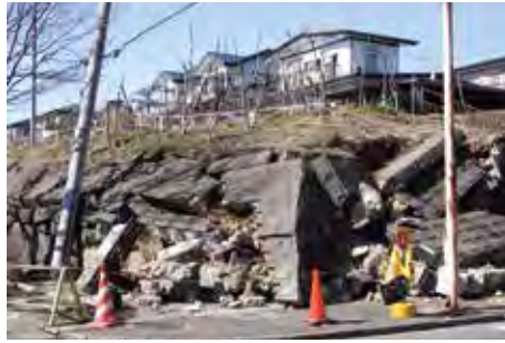
Damage from the earthquake (Hourai neighborhood)
